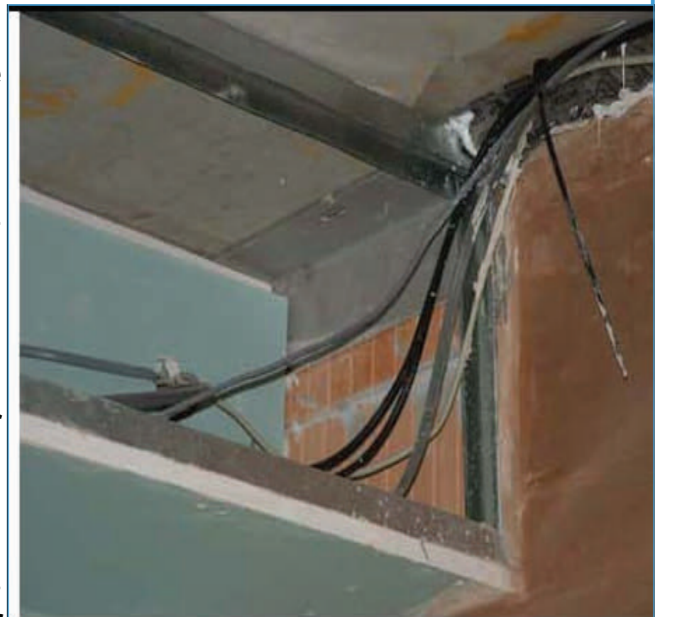
Leakage where section of external wall within services boxing remains unplastered.
