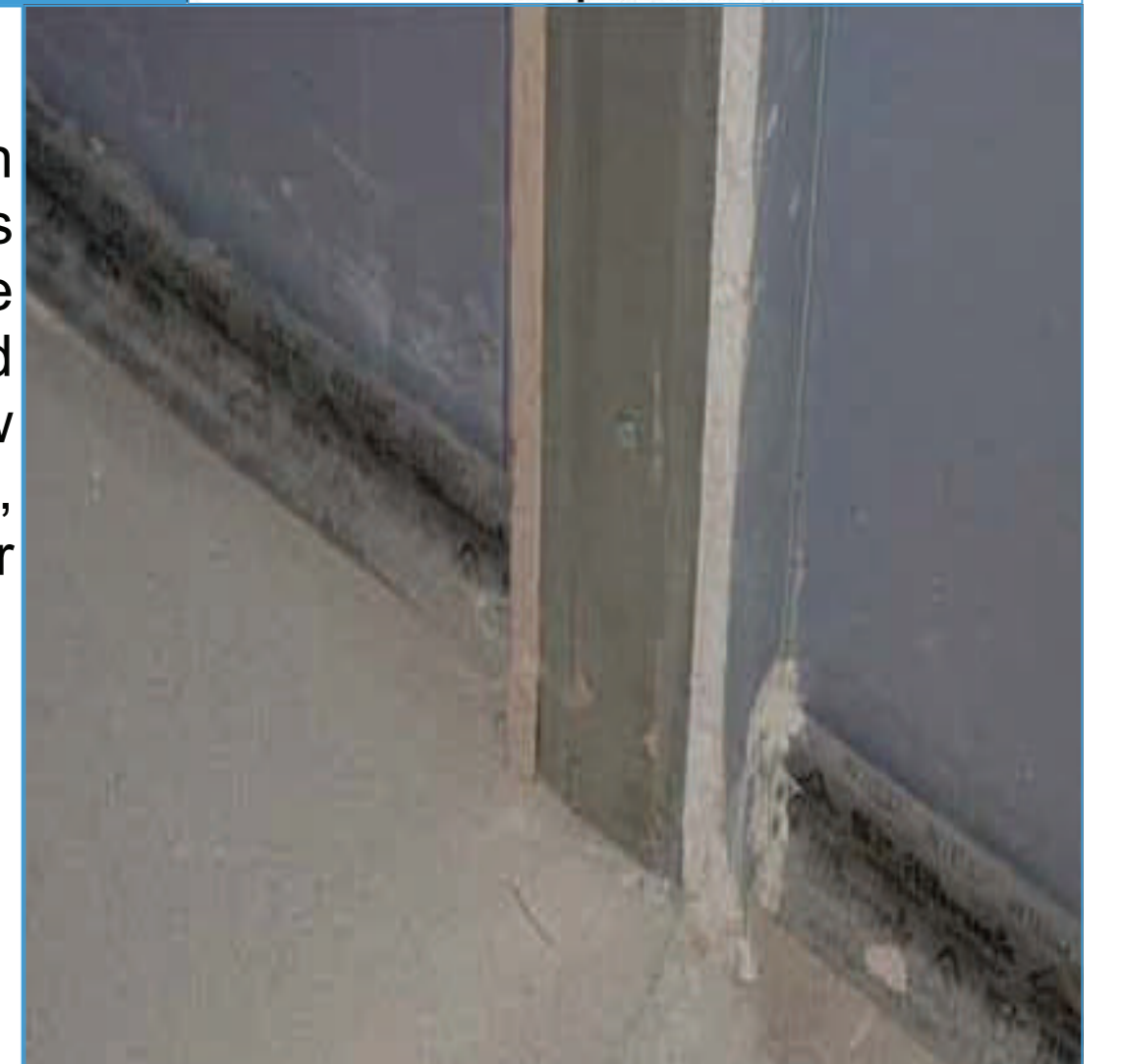
Crack leakage beneath bottom of door frame where membrane seal along base of plaster board is discontinuous.
